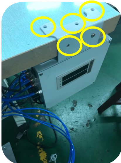
7. 固定控制箱 To fixing the control box
